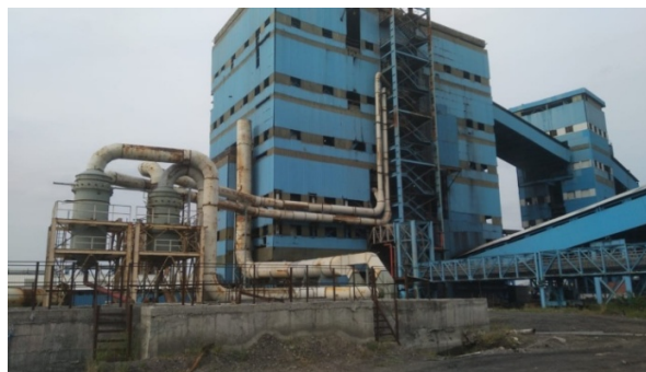
Fig 7: Dust extraction sytem at Coal crusher house
