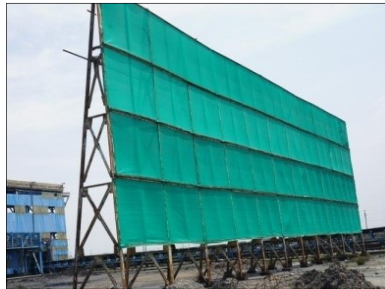
Fig 6: Wind barrier for coal stock yard at NTECL
