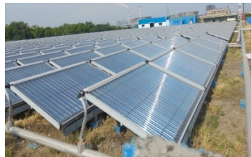
Fig 1: Solar Desalination Plant installed at NTECL
